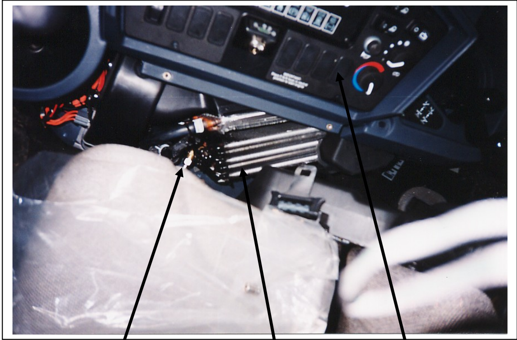
5/16" 90o fitting at expansion valve
